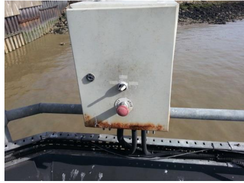
Emergency & Two Way Switch
