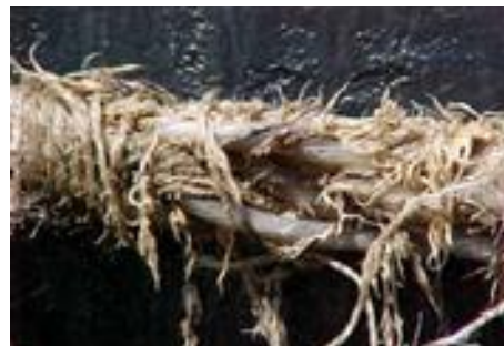
Rope in bad condition
